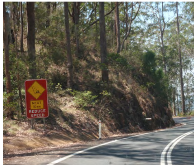
Photograph 1.8: Loose material often falls onto the pavement through the eastern escarpment
