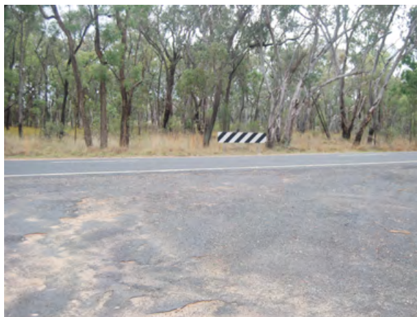
Photograph 3.6: Some road junctions require upgrades
