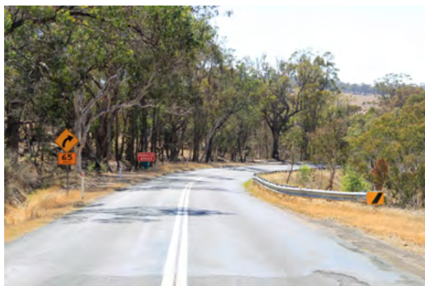
Photograph 3.8: Narrow pavement, no shoulders and tight curves east of the New England Highway
